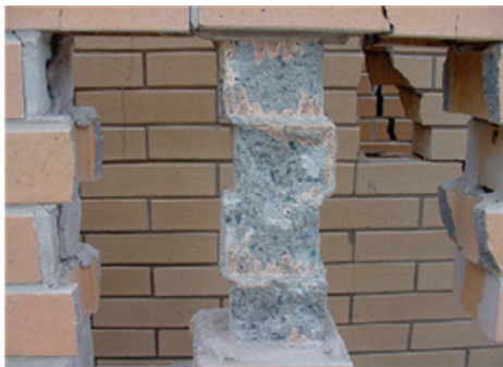
Figure 7. Integrity of typical reinforced grouted core
