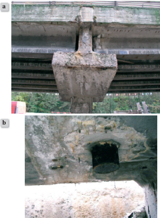
Figure 5. Bridge before repair: a) view of the investigated crosshead in the axis no. 16, b) non-tight collector above the pier cross-beam of bridge
